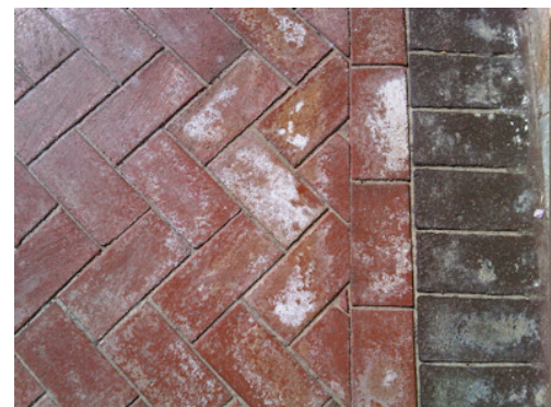
The Wrong Sealer Used on Clay Pavers
