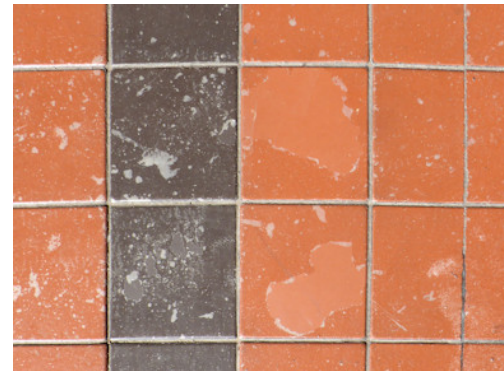
Sealer Popping and Delaminating
