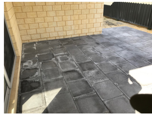
Dangerous Hydrochloric Acids Causes Damage
