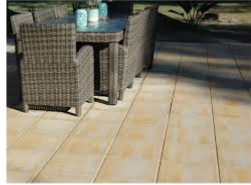
Patchy, Faded & Sealer Turned Yellow
